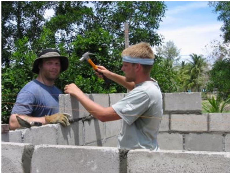
Wave of Hope volunteers crafting the trade of brick laying at Tap Tawan Village.
